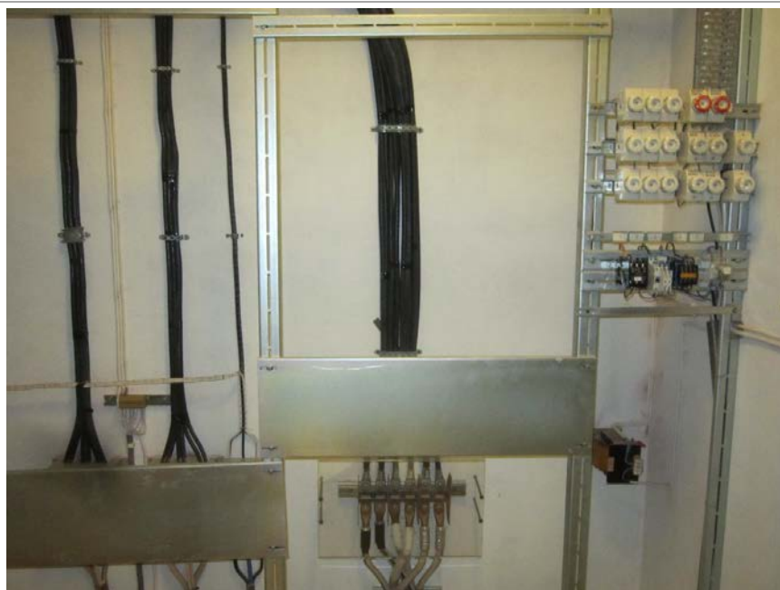
76. Underfordeling D, el-tavle.
