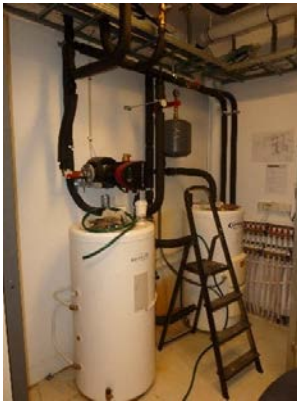
Varmepumpe innedel, fordeling.
